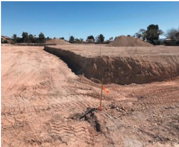
Photo 2. New residential site in Las Vegas, where almost three feet of soil taken from a distant location was used to create a new elevation for both the yard and foundation. The light tan color of the soil indicates low organic content. (Photo by D. Devitt).
