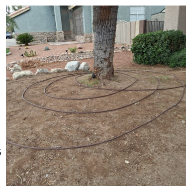
Photos 59 and 60. Drip tubing showing apart and
