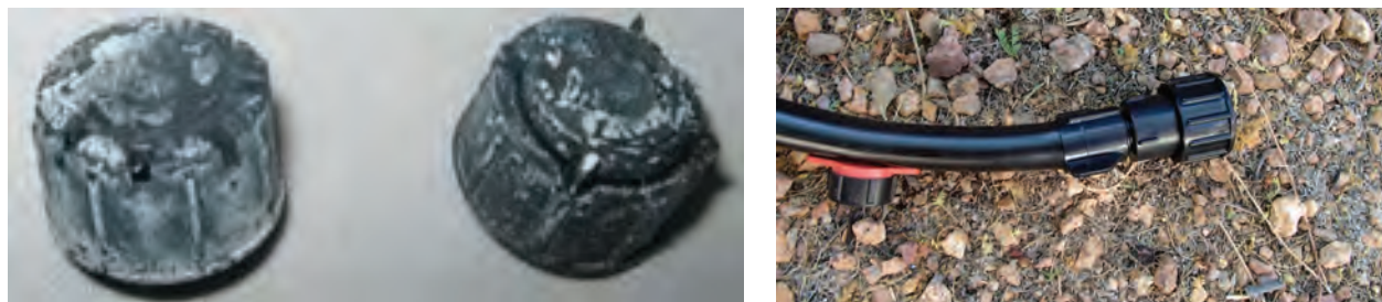
Photos 61 and 62. Salt buildup on drip emitters (left). Plugging might be reduced by flushing the irrigation lines (right) and cleaning the drip filter regularly. (Photos by R. Morris.)
